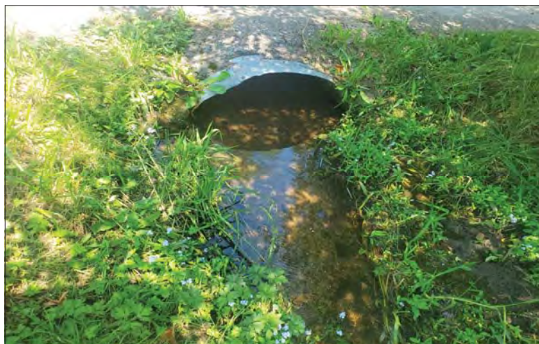
WILLS Saugeen Conservation Filename: 20230704_133445.jpg Photo 22 - October 26, 2023 Durham Creek Flood Plain Mapping Durham Creek: 295 Queen St S Driveway Downstream Face
