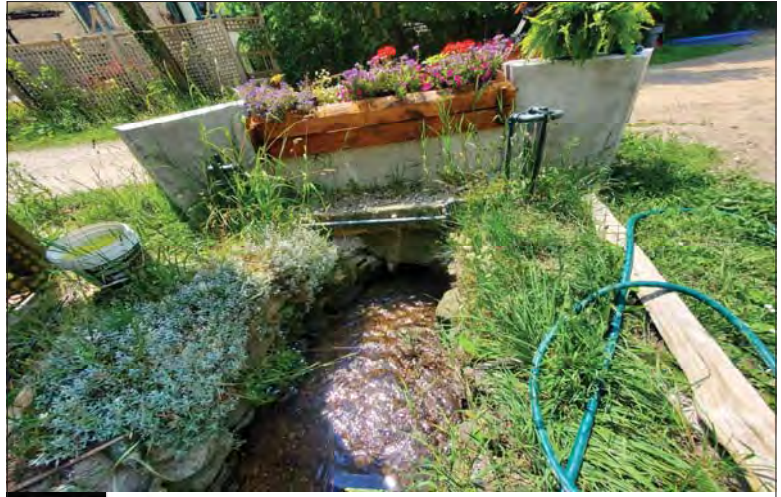
WILLS Saugeen Conservation Filename: 20230705_123005.jpg Photo 68 - October 26, 2023 Durham Creek Flood Plain Mapping Durham Creek: 232 Garafraxa St S Driveway Culvert Upstream Face
