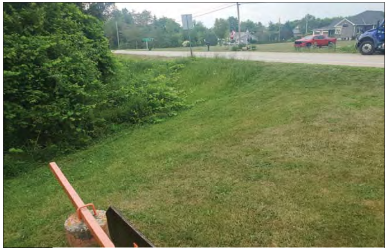
WILLS Saugeen Conservation Filename: 20230706_113948.jpg Photo 344 - October 26, 2023 Durham Creek Flood Plain Mapping Saugeen River: Upper Durham Dam Earth Berm South of Reservoir at End of Berm at Grey County Road 4
