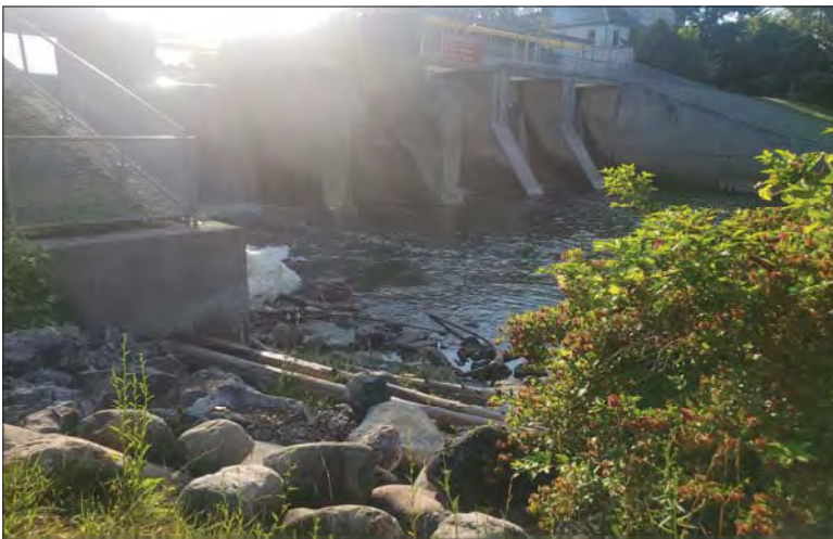
WILLS Saugeen Conservation Filename: 20230707_075420.jpg Photo 245 - October 26, 2023 Durham Creek Flood Plain Mapping Saugeen River: Middle Durham Dam Downstream Face
