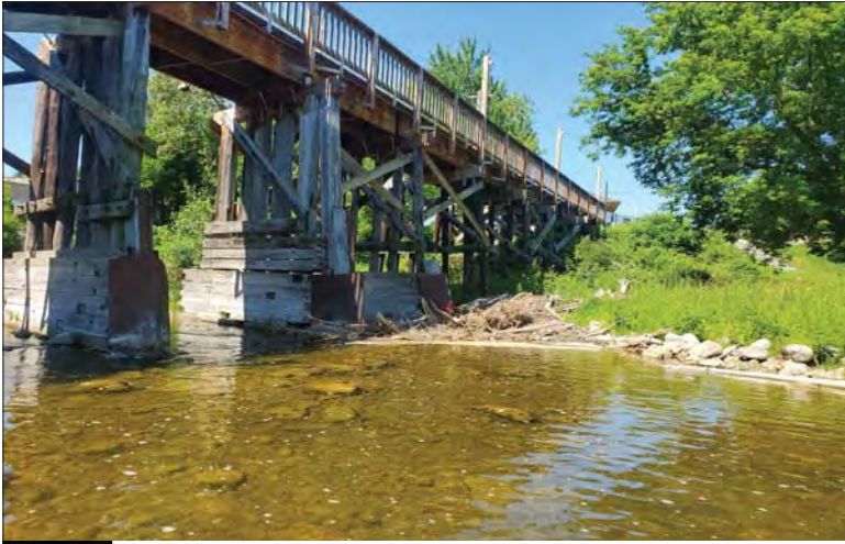
WILLS Saugeen Conservation Filename: 20230707_112808.jpg Photo 229 - October 26, 2023 Durham Creek Flood Plain Mapping Saugeen River: Heritage Walkway Bridge West Bank
