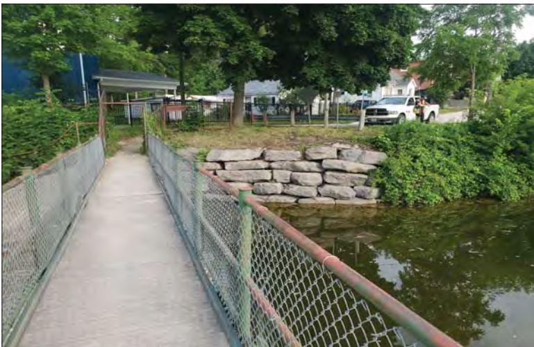
WILLS Saugeen Conservation Filename: 20230706_080109.jpg Photo 131 - October 26, 2023 Durham Creek Flood Plain Mapping Saugeen River: Lower Durham Dam Upstream West Bank
