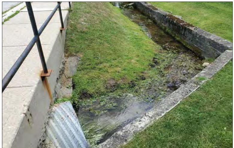
WILLS Saugeen Conservation Filename: 20230705_131239.jpg Photo 82 - October 26, 2023 Durham Creek Flood Plain Mapping Durham Creek: Albert St S Culvert Looking Downstream
