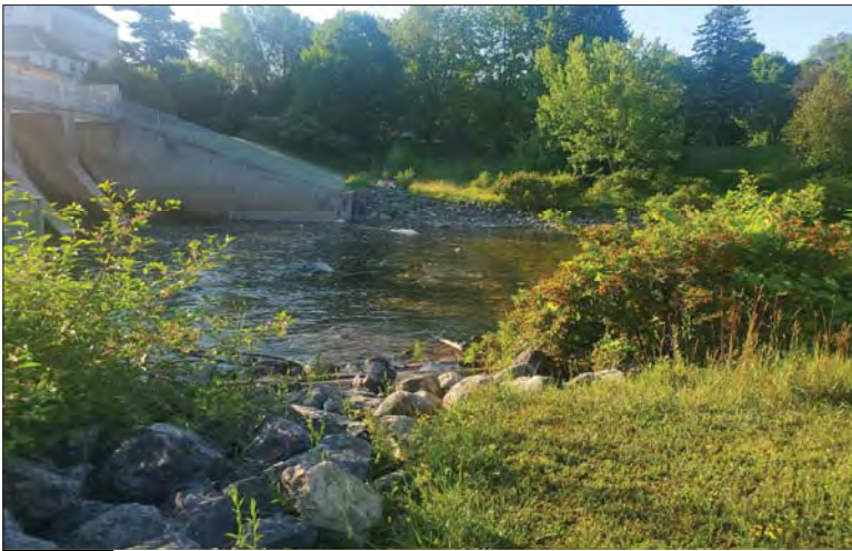
WILLS Saugeen Conservation Filename: 20230707_075439.jpg Photo 247 - October 26, 2023 Durham Creek Flood Plain Mapping Saugeen River: Middle Durham Dam Looking at Downstream South Bank
