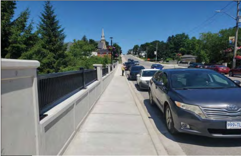
WILLS Saugeen Conservation Filename: 20230707_122940.jpg Photo 199 - October 26, 2023 Durham Creek Flood Plain Mapping Saugen River: Highway 6 Bridge South Abutment Looking North
