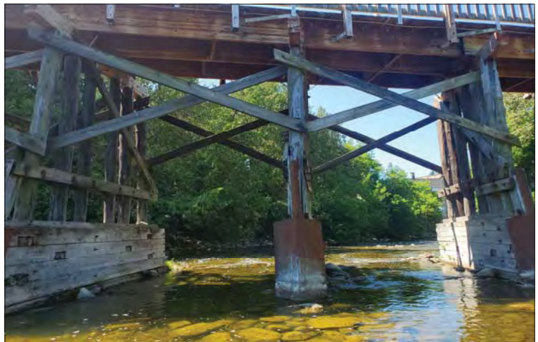
WILLS Saugeen Conservation Filename: 20230707_112804.jpg Photo 228 - October 26, 2023 Durham Creek Flood Plain Mapping Saugeen River: Heritage Walkway Bridge Piers
