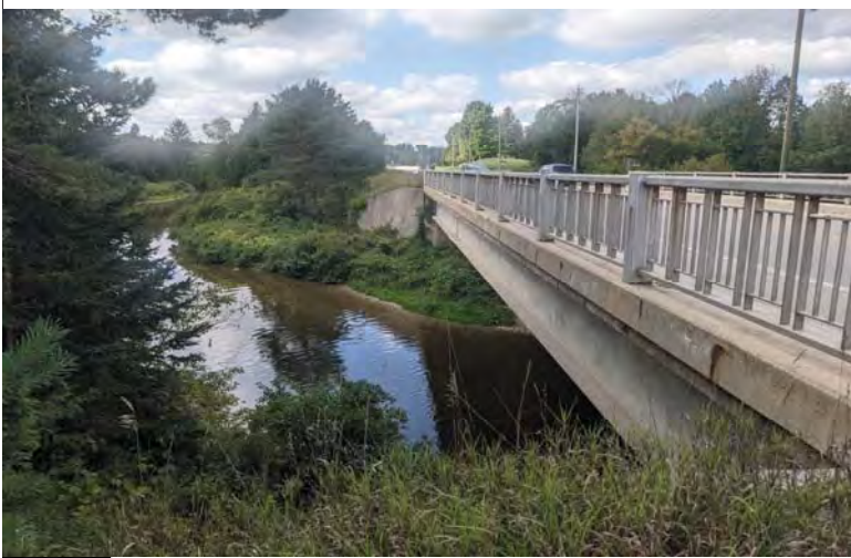
WILLS Saugeen Conservation Filename: PXL_20230914_161914005.jpg Photo 1 - September 14, 2023 Durham Creek Flood Plain Mapping Saugeen River: Grey County Road 4 Bridge Upstream Face
