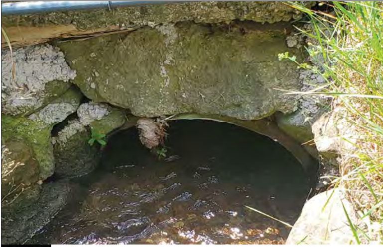
WILLS Saugeen Conservation Filename: 20230705_123001.jpg Photo 67 - October 26, 2023 Durham Creek Flood Plain Mapping Durham Creek: 232 Garafraxa St S Driveway Culvert Upstream Face
