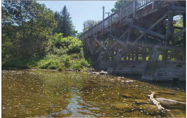
WILLS Saugeen Conservation Filename: 20230707_112812.jpg Photo 230 - October 26, 2023 Durham Creek Flood Plain Mapping Saugeen River: Heritage Walkway Bridge East Bank
