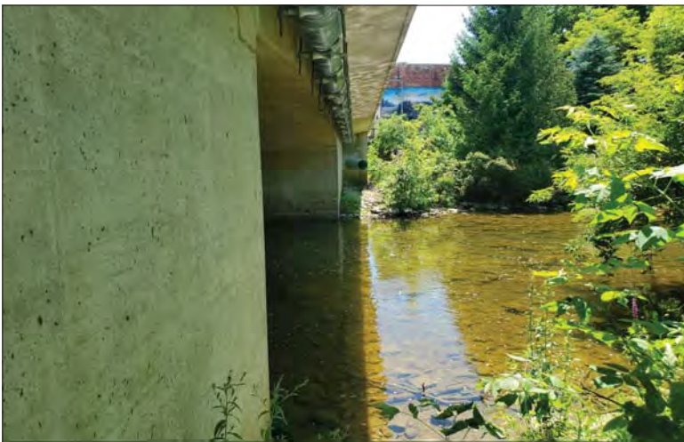
WILLS Saugeen Conservation Filename: 20230707_133940.jpg Photo 203 - October 26, 2023 Durham Creek Flood Plain Mapping Saugen River: Highway 6 Bridge Downstream Opening
