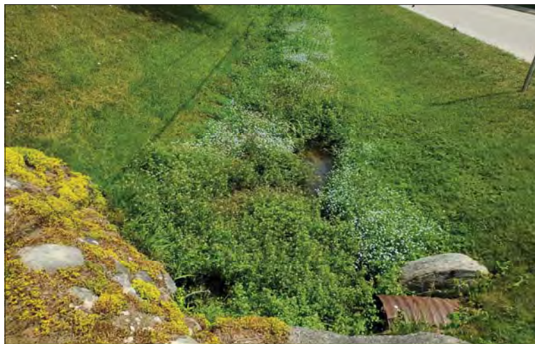
WILLS Saugeen Conservation Filename: 20230705_131944.jpg Photo 86 - October 26, 2023 Durham Creek Flood Plain Mapping Durham Creek: Saddler St E Culvert Looking Upstream
