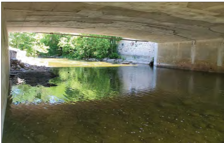
WILLS Saugeen Conservation Filename: 20230707_134007.jpg Photo 205 - October 26, 2023 Durham Creek Flood Plain Mapping Saugeen River: Highway 6 Bridge Soffit Looking Upstream
