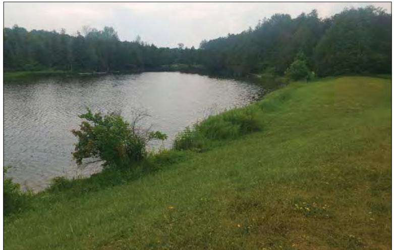
WILLS Saugeen Conservation Filename: 20230706_113318.jpg Photo 334 - October 26, 2023 Durham Creek Flood Plain Mapping Saugeen River: Upper Durham Dam View from Earth Berm
