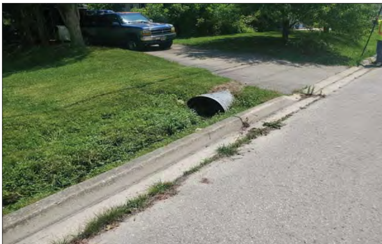
WILLS Saugeen Conservation Filename: 20230704_133408.jpg Photo 19 - October 26, 2023 Durham Creek Flood Plain Mapping Durham Creek: 295 Queen St S Driveway Upstream Face
