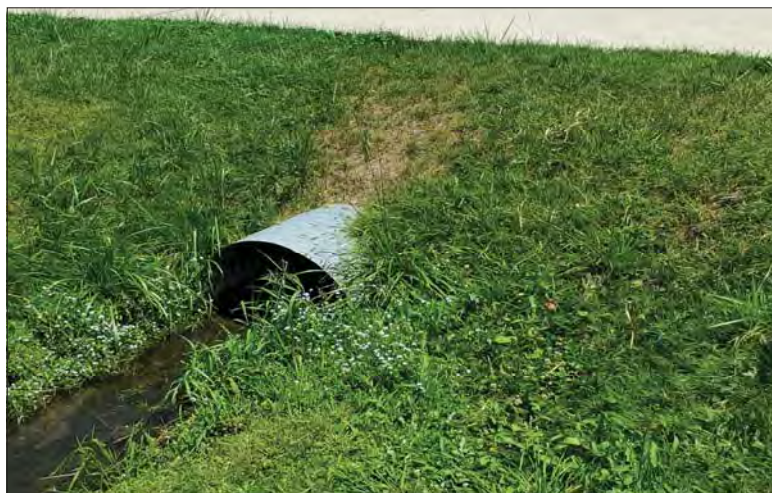
WILLS Saugeen Conservation Filename: 20230704_125833.jpg Photo 10 - October 26, 2023 Durham Creek Flood Plain Mapping Durham Creek: 274 South St W Driveway Downstream Face
