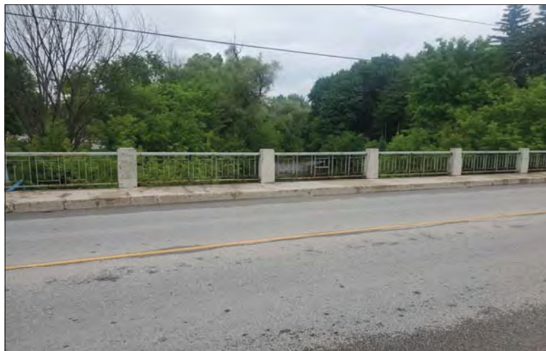
WILLS Saugeen Conservation Filename: 20230706_154214.jpg Photo 182 - October 26, 2023 Durham Creek Flood Plain Mapping Saugeen River: Lambton St E Bridge Looking North
