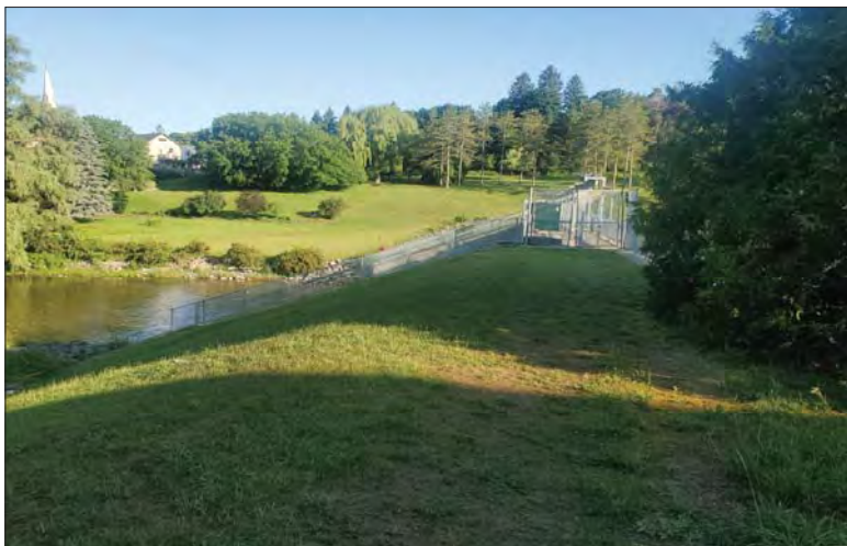
WILLS Saugeen Conservation Filename: 20230707_075933.jpg Photo 271 - October 26, 2023 Durham Creek Flood Plain Mapping Saugeen River: Middle Durham Dam Looking Northwest
