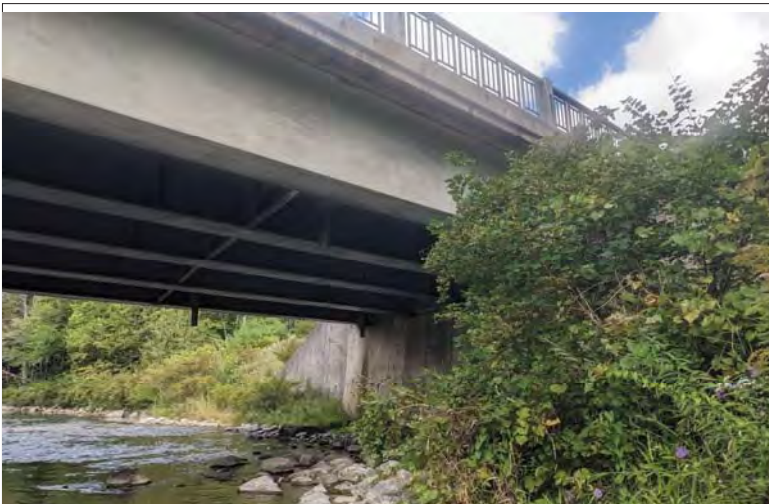
WILLS Saugeen Conservation Filename: PXL_20230914_161831636.jpg Photo 3 - September 14, 2023 Durham Creek Flood Plain Mapping Saugeen River: Grey County Road 4 Bridge Upstream Soffit and East Abutment
