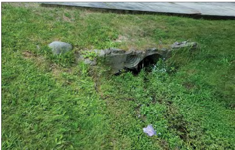
WILLS Saugeen Conservation Filename: 20230705_133928.jpg Photo 91 - October 26, 2023 Durham Creek Flood Plain Mapping Durham Creek: 242 Saddler St E Driveway Culvert Upstream Face
