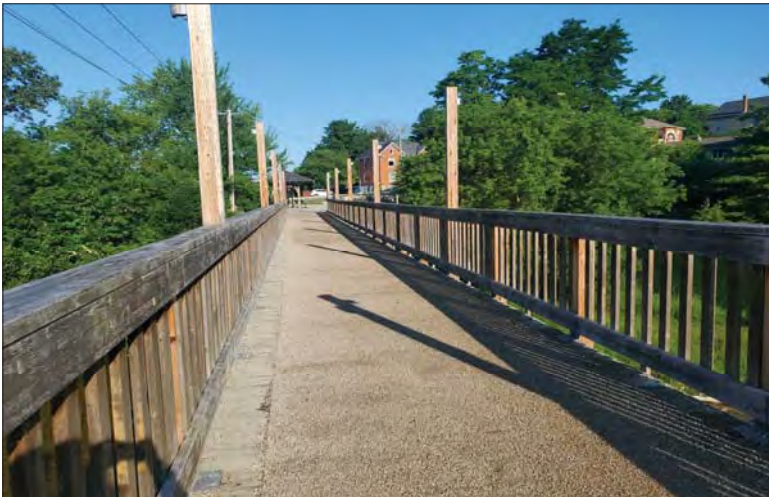
WILLS Saugeen Conservation Filename: 20230707_081613.jpg Photo 219 - October 26, 2023 Durham Creek Flood Plain Mapping Saugeen River: Heritage Walkway Bridge Deck Looking West
