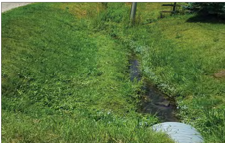
WILLS Saugeen Conservation Filename: 20230704_125815.jpg Photo 9 - October 26, 2023 Durham Creek Flood Plain Mapping Durham Creek: 274 South St W Driveway Facing Downstream
