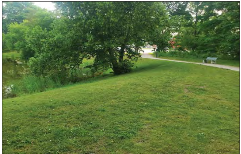
WILLS Saugeen Conservation Filename: 20230706_080411.jpg Photo 158 - October 26, 2023 Durham Creek Flood Plain Mapping Saugeen River: Lower Durham Dam East End of Earth Berm
