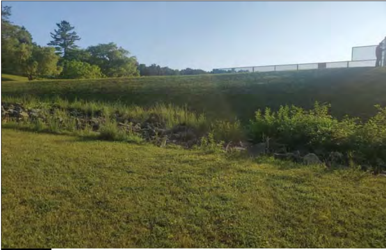
WILLS Saugeen Conservation Filename: 20230707_075358.jpg Photo 241 - October 26, 2023 Durham Creek Flood Plain Mapping Saugeen River: Middle Durham Dam Downstream of Dam Looking North
