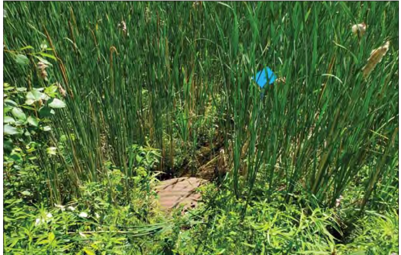
WILLS Saugeen Conservation Filename: 20230707_143944.jpg Photo 118 - October 26, 2023 Durham Creek Flood Plain Mapping Durham Creek: Grey County Rd 4 Culvert Downstream Outlet
