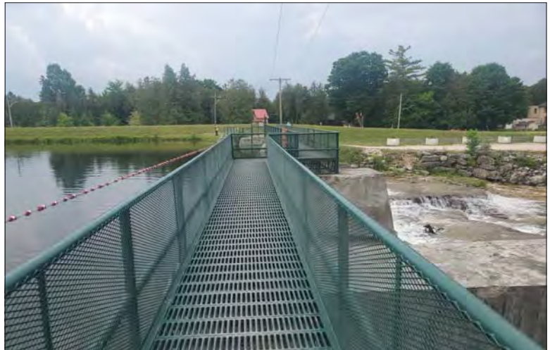
WILLS Saugeen Conservation Filename: 20230706_111850.jpg Photo 304 - October 26, 2023 Durham Creek Flood Plain Mapping Saugeen River: Upper Durham Dam Deck Looking South
