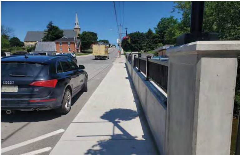
WILLS Saugeen Conservation Filename: 20230707_122842.jpg Photo 201 - October 26, 2023 Durham Creek Flood Plain Mapping Saugen River: Highway 6 Bridge South Abutment Looking North
