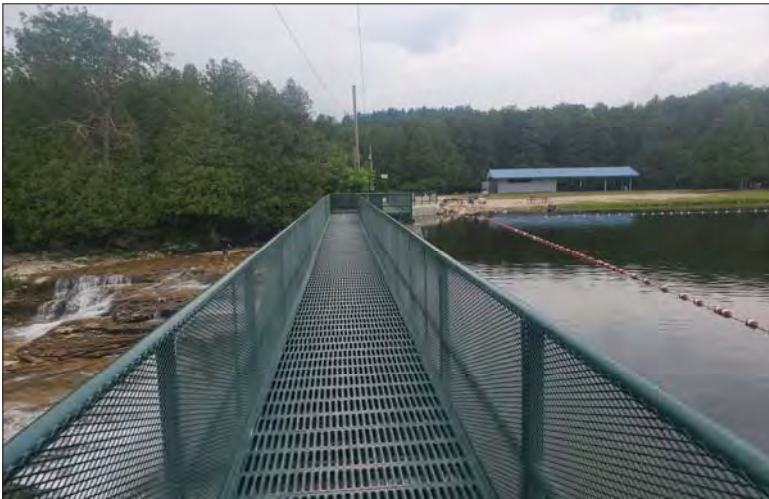
WILLS Saugeen Conservation Filename: 20230706_111641.jpg Photo 291 - October 26, 2023 Durham Creek Flood Plain Mapping Saugeen River: Upper Durham Dam Deck
