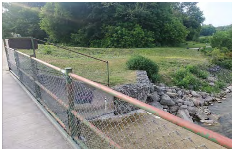
WILLS Saugeen Conservation Filename: 20230706_080206.jpg Photo 140 - October 26, 2023 Durham Creek Flood Plain Mapping Saugeen River: Lower Durham Dam Downstream East Bank
