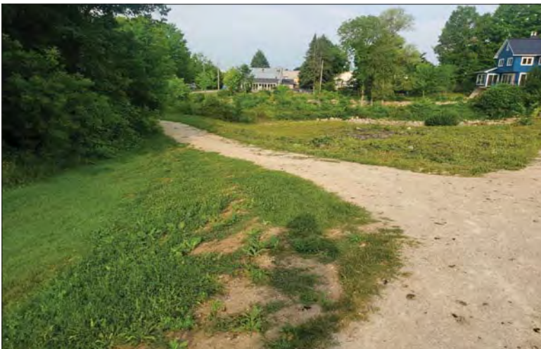
WILLS Saugeen Conservation Filename: 20230706_080331.jpg Photo 155 - October 26, 2023 Durham Creek Flood Plain Mapping Saugeen River: Lower Durham Dam Emergency Spillway
