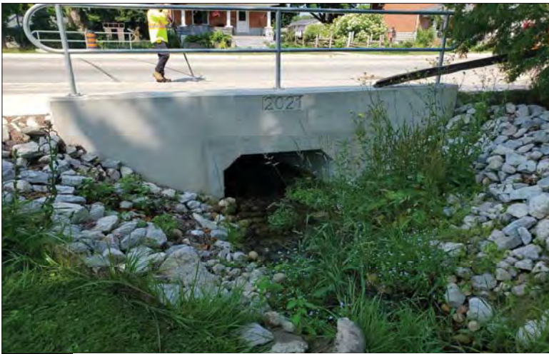
WILLS Saugeen Conservation Filename: 20230705_112443.jpg Photo 61 - October 26, 2023 Durham Creek Flood Plain Mapping Durham Creek: Garafraxa St S Culvert Upstream Face
