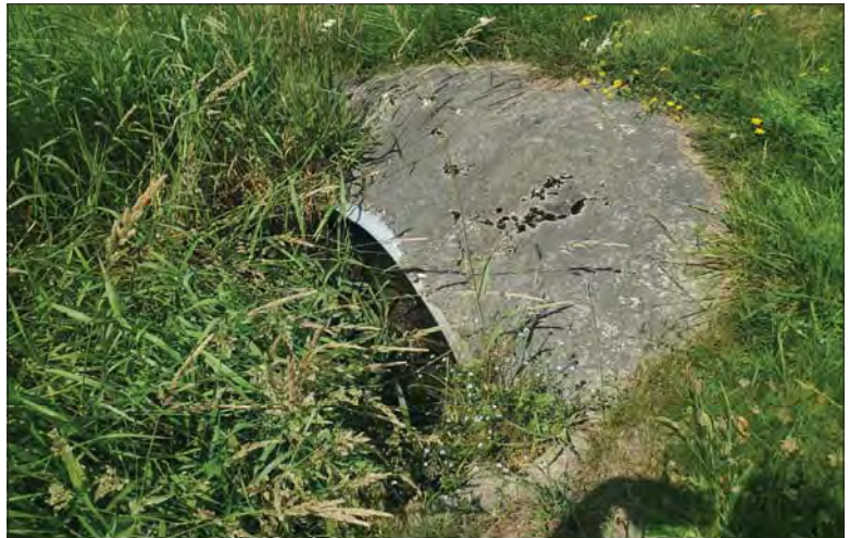
WILLS Saugeen Conservation Filename: 20230705_145718.jpg Photo 100 - October 26, 2023 Durham Creek Flood Plain Mapping Durham Creek: Elgin St S Culvert Downstream Face
