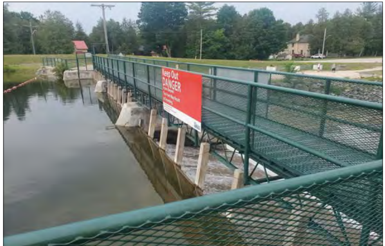
WILLS Saugeen Conservation Filename: 20230706_111747.jpg Photo 298 - October 26, 2023 Durham Creek Flood Plain Mapping Saugeen River: Upper Durham Dam Upstream Face
