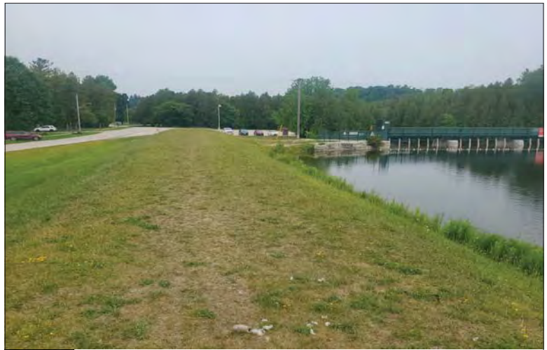
WILLS Saugeen Conservation Filename: 20230706_113211.jpg Photo 326 - October 26, 2023 Durham Creek Flood Plain Mapping Saugeen River: Upper Durham Dam Earth Berm
