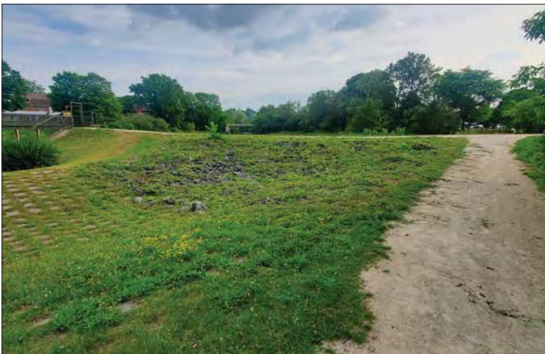
WILLS Saugeen Conservation Filename: 20230706_080843.jpg Photo 149 - October 26, 2023 Durham Creek Flood Plain Mapping Saugeen River: Lower Durham Dam Emergency Spillway
