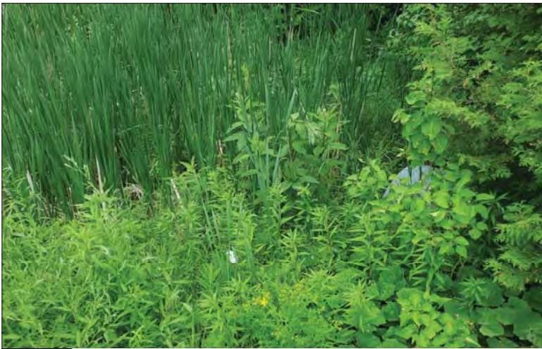
WILLS Saugeen Conservation Filename: 20230705_162635.jpg Photo 109 - October 26, 2023 Durham Creek Flood Plain Mapping Durham Creek: 479 Lambton St E Driveway Culvert Upstream End
