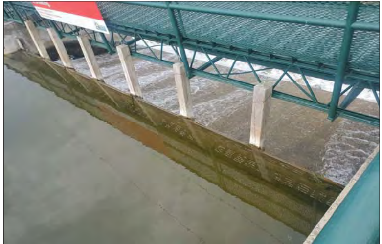
WILLS Saugeen Conservation Filename: 20230706_111805.jpg Photo 300 - October 26, 2023 Durham Creek Flood Plain Mapping Saugeen River: Upper Durham Dam Upstream Face of Middle Spillway
