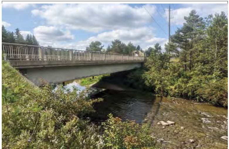
WILLS Saugeen Conservation Filename: PXL_20230914_162306638.MP.jpg Photo 10 - September 14, 2023 Durham Creek Flood Plain Mapping Saugeen River: Grey County Road 4 Bridge Downstream Face
