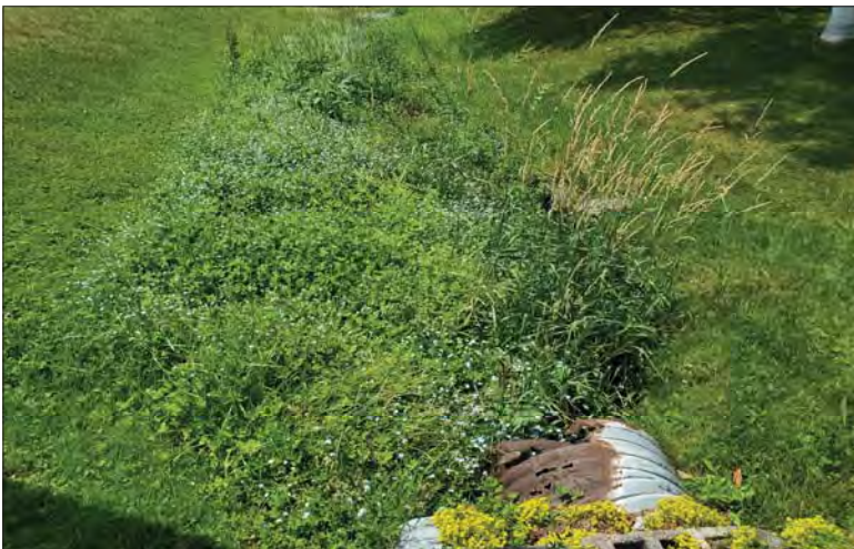
WILLS Saugeen Conservation Filename: 20230705_133951.jpg Photo 93 - October 26, 2023 Durham Creek Flood Plain Mapping Durham Creek: 242 Saddler St E Driveway Culvert Looking Downstream
