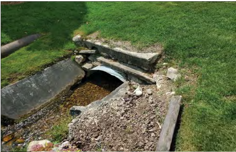
WILLS Saugeen Conservation Filename: 20230705_131203.jpg Photo 79 - October 26, 2023 Durham Creek Flood Plain Mapping Durham Creek: Albert St S Culvert Upstream Face
