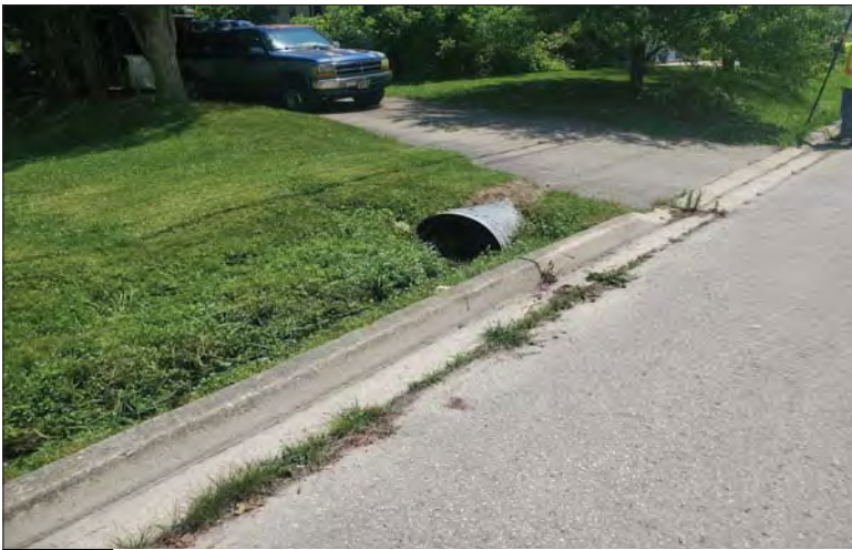
WILLS Saugeen Conservation Filename: 20230704_133408.jpg Photo 19 - October 26, 2023 Durham Creek Flood Plain Mapping Durham Creek: 295 Queen St S Driveway Upstream Face
