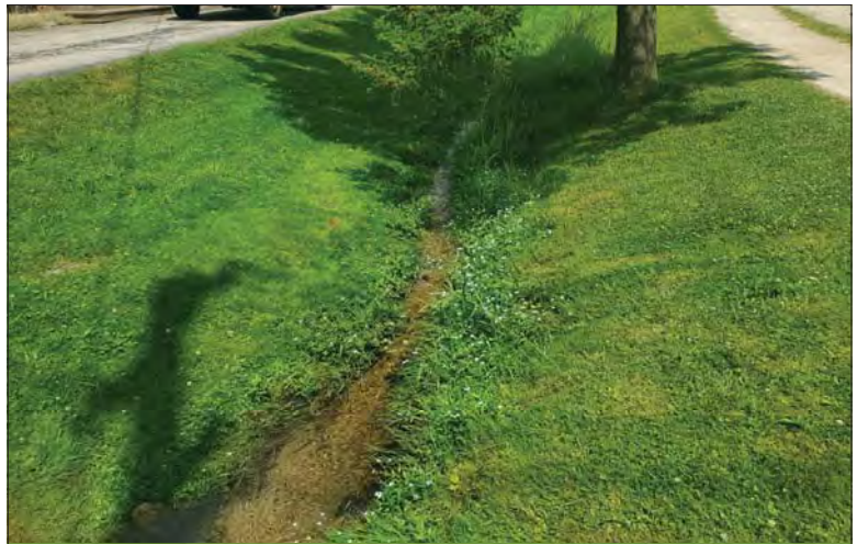
WILLS Saugeen Conservation Filename: 20230705_145634.jpg Photo 98 - October 26, 2023 Durham Creek Flood Plain Mapping Durham Creek: Elgin St S Culvert Looking Upstream
