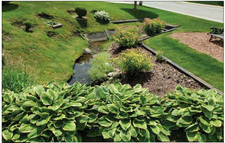
WILLS Saugeen Conservation Filename: 20230705_132043.jpg Photo 88 - October 26, 2023 Durham Creek Flood Plain Mapping Durham Creek: Saddler St E Culvert Looking Downstream
