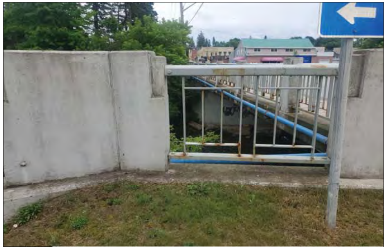
WILLS Saugeen Conservation Filename: 20230706_154405.jpg Photo 176 - October 26, 2023 Durham Creek Flood Plain Mapping Saugeen River: Lambton St E Bridge Upstream Face and West Wingwall
