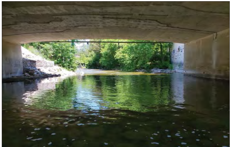
WILLS Saugeen Conservation Filename: 20230707_134142.jpg Photo 206 - October 26, 2023 Durham Creek Flood Plain Mapping Saugeen River: Highway 6 Bridge Soffit Looking Upstream
