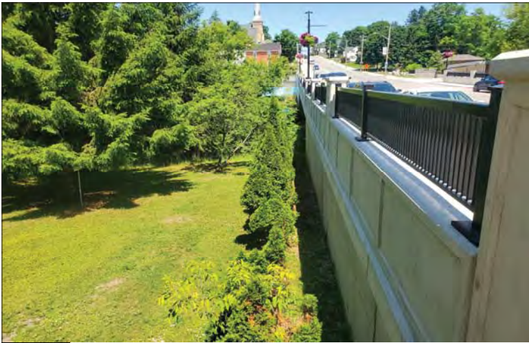
WILLS Saugeen Conservation Filename: 20230707_122929.jpg Photo 191 - October 26, 2023 Durham Creek Flood Plain Mapping Saugeen River: Highway 6 Bridge Downstream Face
