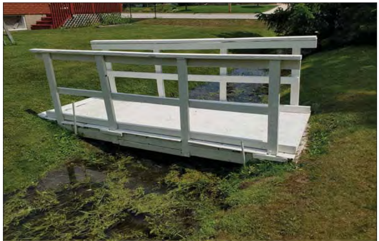
WILLS Saugeen Conservation Filename: 20230705_131104.jpg Photo 76 - October 26, 2023 Durham Creek Flood Plain Mapping Durham Creek: 197 Saddler St E Backyard Footbridge Downstream Face
