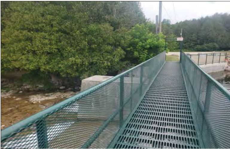
WILLS Saugeen Conservation Filename: 20230706_111755.jpg Photo 299 - October 26, 2023 Durham Creek Flood Plain Mapping Saugeen River: Upper Durham Dam Deck Looking North
