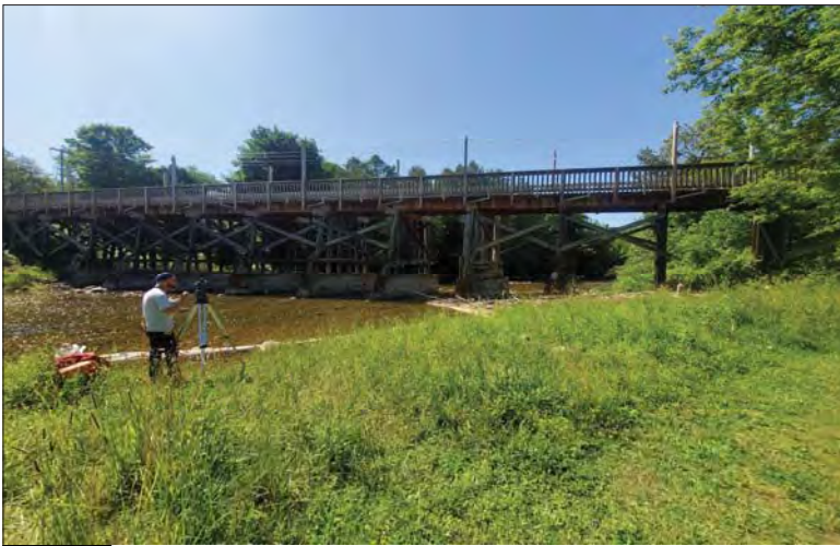
WILLS Saugeen Conservation Filename: 20230707_105916.jpg Photo 211 - October 26, 2023 Durham Creek Flood Plain Mapping Saugeen River: Heritage Walkway Bridge Upstream Face
