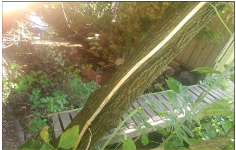
WILLS Saugeen Conservation Filename: 20230704_155826.jpg Photo 26 - October 26, 2023 Durham Creek Flood Plain Mapping Durham Creek: 269 Queen St S Backyard Footbridge
