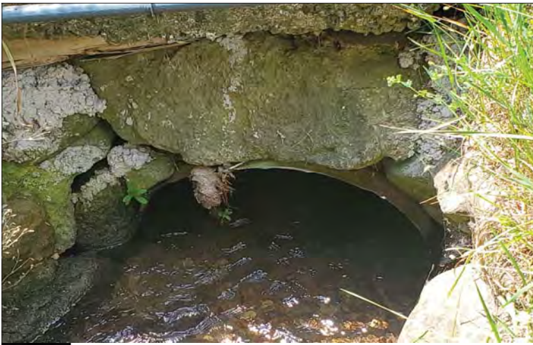
WILLS Saugeen Conservation Filename: 20230705_123001.jpg Photo 67 - October 26, 2023 Durham Creek Flood Plain Mapping Durham Creek: 232 Garafraxa St S Driveway Culvert Upstream Face
