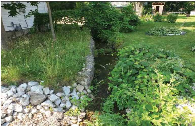
WILLS Saugeen Conservation Filename: 20230705_112558.jpg Photo 63 - October 26, 2023 Durham Creek Flood Plain Mapping Durham Creek: Garafraxa St S Culvert Looking Downstream
