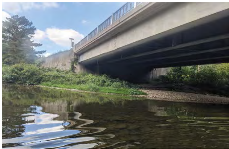
WILLS Saugeen Conservation Filename: PXL_20230914_161825667.jpg Photo 2 - September 14, 2023 Durham Creek Flood Plain Mapping Saugeen River: Grey County Road 4 Bridge Upstream Soffit and West Wingwall
