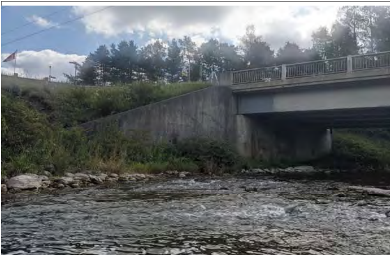
WILLS Saugeen Conservation Filename: PXL_20230914_161730650.jpg Photo 5 - September 14, 2023 Durham Creek Flood Plain Mapping Saugeen River: Grey County Road 4 Bridge Downstream West Wingwall
