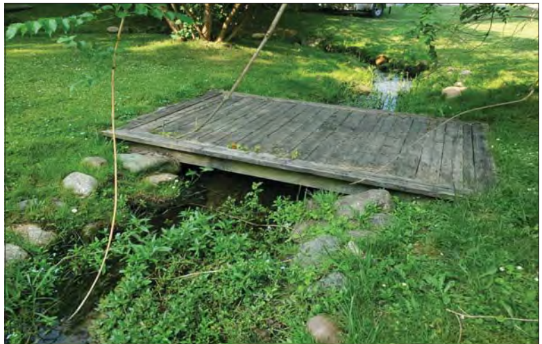
WILLS Saugeen Conservation Filename: 20230705_092733.jpg Photo 38 - October 26, 2023 Durham Creek Flood Plain Mapping Durham Creek: 249 Queen St S Backyard Footbridge 1 Upstream Face
