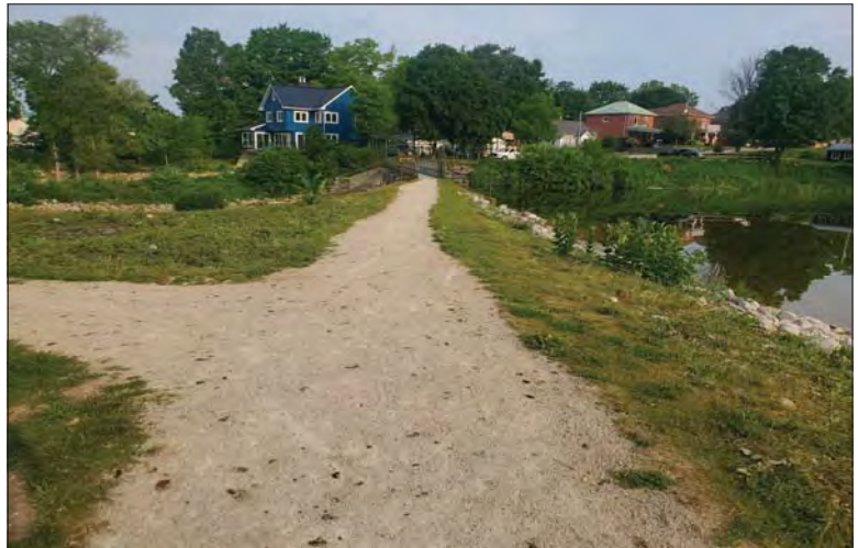
WILLS Saugeen Conservation Filename: 20230706_080328.jpg Photo 154 - October 26, 2023 Durham Creek Flood Plain Mapping Saugeen River: Lower Durham Dam Earth Berm and Emergency Spillway
