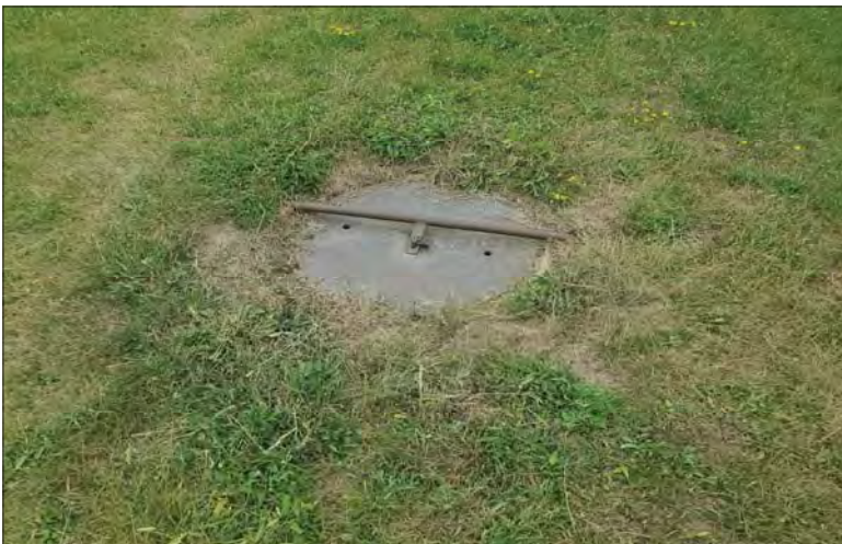
WILLS Saugeen Conservation Filename: 20230706_113355.jpg Photo 335 - October 26, 2023 Durham Creek Flood Plain Mapping Saugeen River: Upper Durham Dam Earthen Berm Cover Plate
