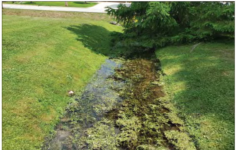
WILLS Saugeen Conservation Filename: 20230705_131047.jpg Photo 74 - October 26, 2023 Durham Creek Flood Plain Mapping Durham Creek: 197 Saddler St E Backyard Footbridge Looking Upstream
