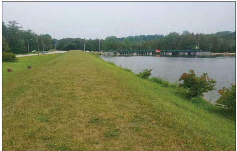
WILLS Saugeen Conservation Filename: 20230706_113312.jpg Photo 332 - October 26, 2023 Durham Creek Flood Plain Mapping Saugeen River: Upper Durham Dam Earth Berm
