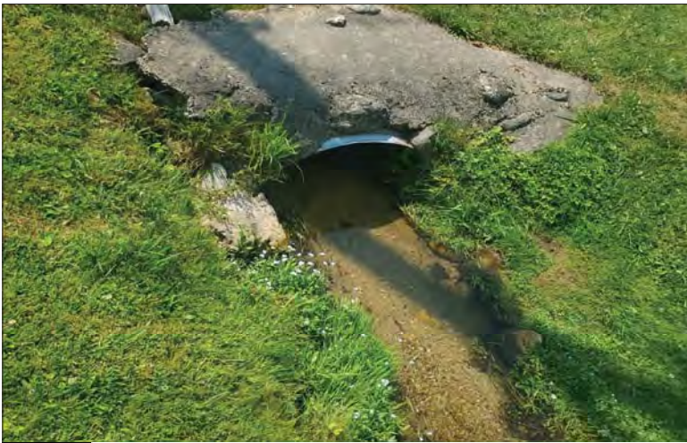
WILLS Saugeen Conservation Filename: 20230705_145625.jpg Photo 97 - October 26, 2023 Durham Creek Flood Plain Mapping Durham Creek: Elgin St S Culvert Upstream Face
