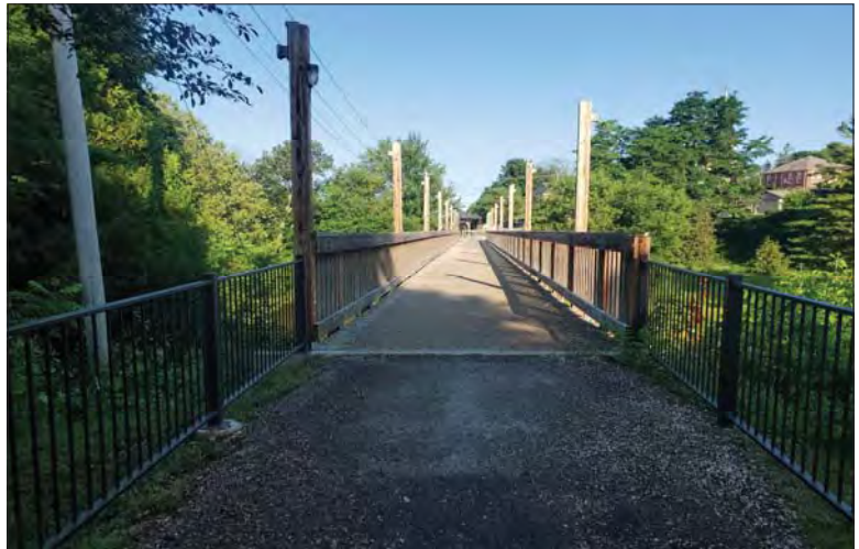
WILLS Saugeen Conservation Filename: 20230707_081519.jpg Photo 214 - October 26, 2023 Durham Creek Flood Plain Mapping Saugeen River: Heritage Walkway Bridge East Abutment Looking West
