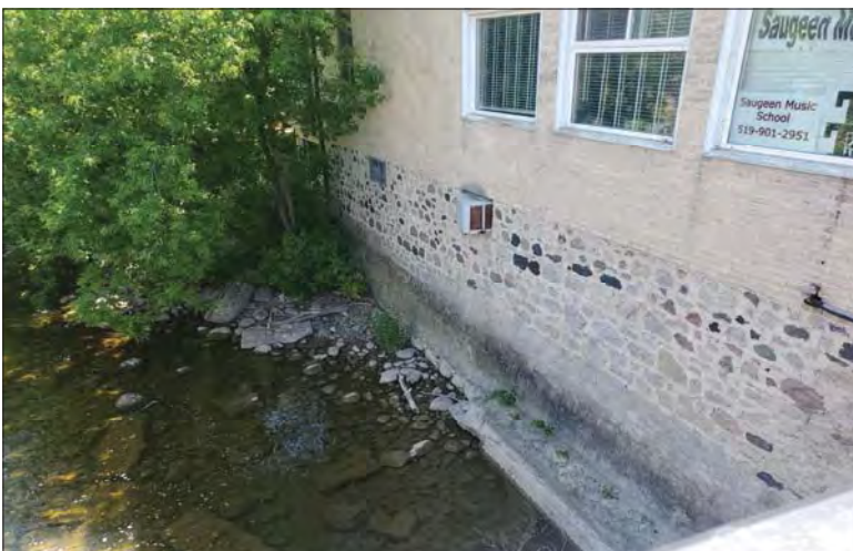
WILLS Saugeen Conservation Filename: 20230707_122805.jpg Photo 197 - October 26, 2023 Durham Creek Flood Plain Mapping Saugeen River: Highway 6 Bridge Upstream South Bank
