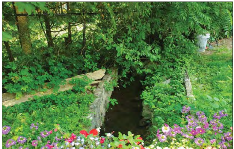
WILLS Saugeen Conservation Filename: 20230705_123026.jpg Photo 70 - October 26, 2023 Durham Creek Flood Plain Mapping Durham Creek: 232 Garafraxa St S Driveway Culvert Looking Downstream
