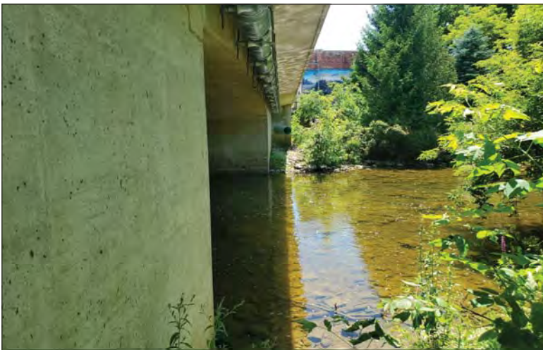
WILLS Saugeen Conservation Filename: 20230707_133940.jpg Photo 203 - October 26, 2023 Durham Creek Flood Plain Mapping Saugeen River: Highway 6 Bridge Downstream Opening
