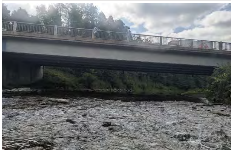
WILLS Saugeen Conservation Filename: PXL_20230914_161732619.jpg Photo 6 - September 14, 2023 Durham Creek Flood Plain Mapping Saugeen River: Grey County Road 4 Bridge Downstream Face
