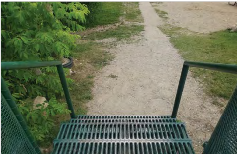
WILLS Saugeen Conservation Filename: 20230706_111902.jpg Photo 305 - October 26, 2023 Durham Creek Flood Plain Mapping Saugeen River: Upper Durham Dam Deck Stairs North Side
