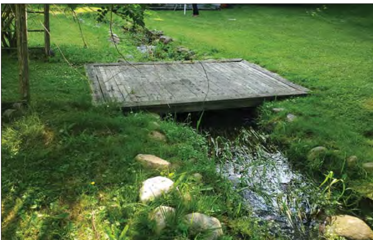
WILLS Saugeen Conservation Filename: 20230705_092802.jpg Photo 41 - October 26, 2023 Durham Creek Flood Plain Mapping Durham Creek: 249 Queen St S Backyard Footbridge 1 Downstream Face
