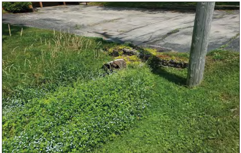
WILLS Saugeen Conservation Filename: 20230705_134004.jpg Photo 94 - October 26, 2023 Durham Creek Flood Plain Mapping Durham Creek: 242 Saddler St E Driveway Culvert Downstream Face
