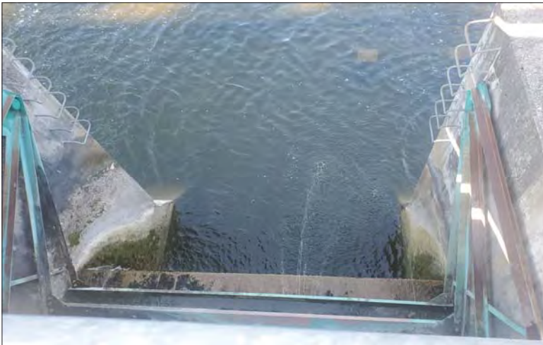
WILLS Saugeen Conservation Filename: 20230707_075734.jpg Photo 255 - October 26, 2023 Durham Creek Flood Plain Mapping Saugeen River: Middle Durham Dam Sluice Gate
